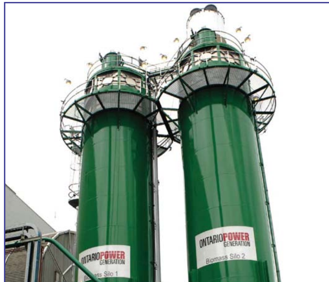
Biomass towers at OPG's Nanticoke GS
